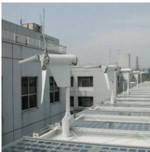
Proven Energy 2.5kW turbine rooftop array
