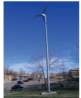
Skystream 1.8kW turbine
