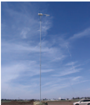
Guyed Monopole Tower
