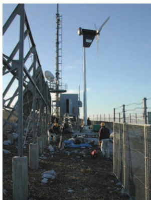
Proven Energy 6kW turbine powering telecommunications equipment
