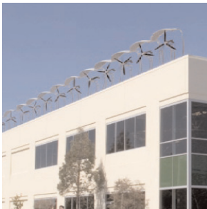
AeroVironment rooftop array
