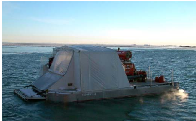
Figure 4.12 Working platform with heated enclosure to avoid icing and freezing of equipment.
