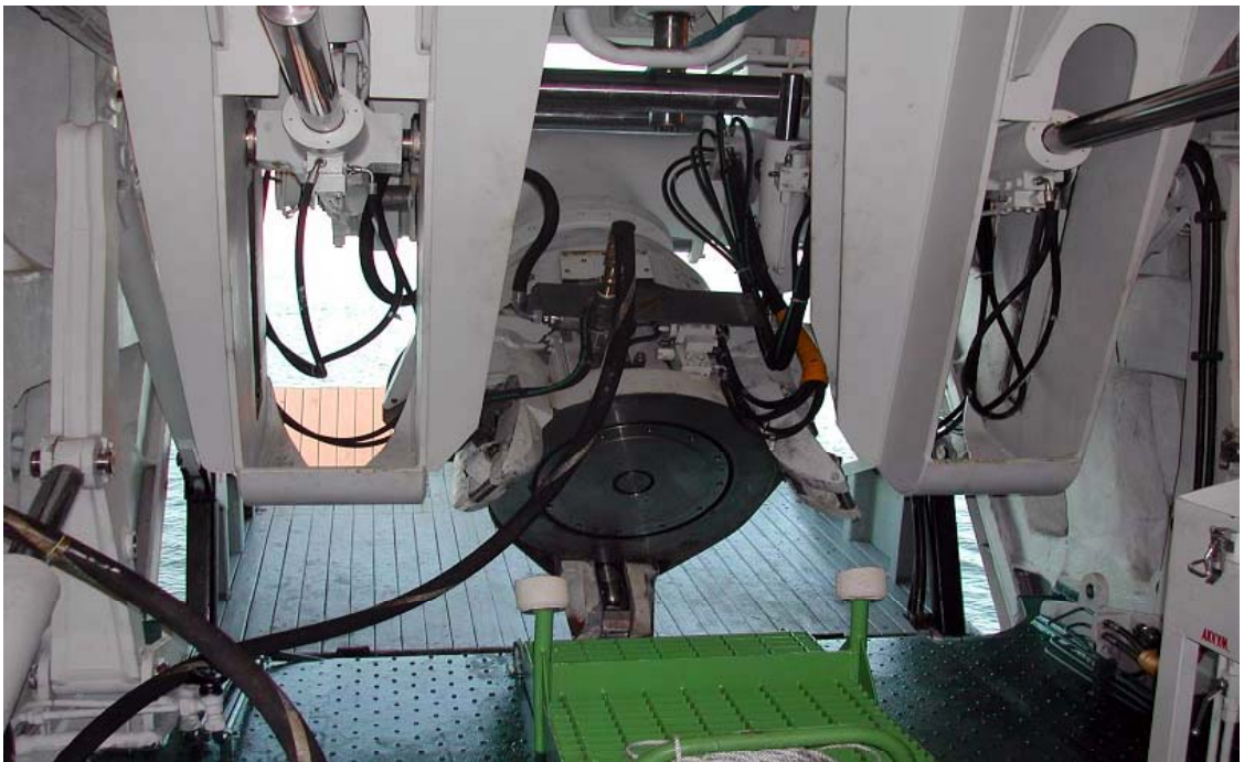
MT "Saratov" – Bow Loading System manifold
