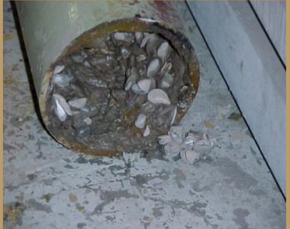
Water Cooled Transformer Piping
