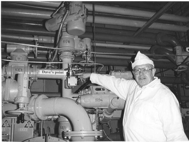
Real-time monitoring equipment is installed at this point where a pipe carrying 90% enriched gas meets a pipe carrying 1.5% enriched uranium gas to produce 4.4% enriched uranium for the U.S.-Russian HEU Purchase agreement. (The blend point is labeled “Dave’s point” after one of the U.S. designers of the equipment, shown in the photo.) The United States should offer to pay Russia to drastically accelerate this blend-down, with the goal of eliminating the proliferation risk posed by excess HEU within a few years. Source: DOE
